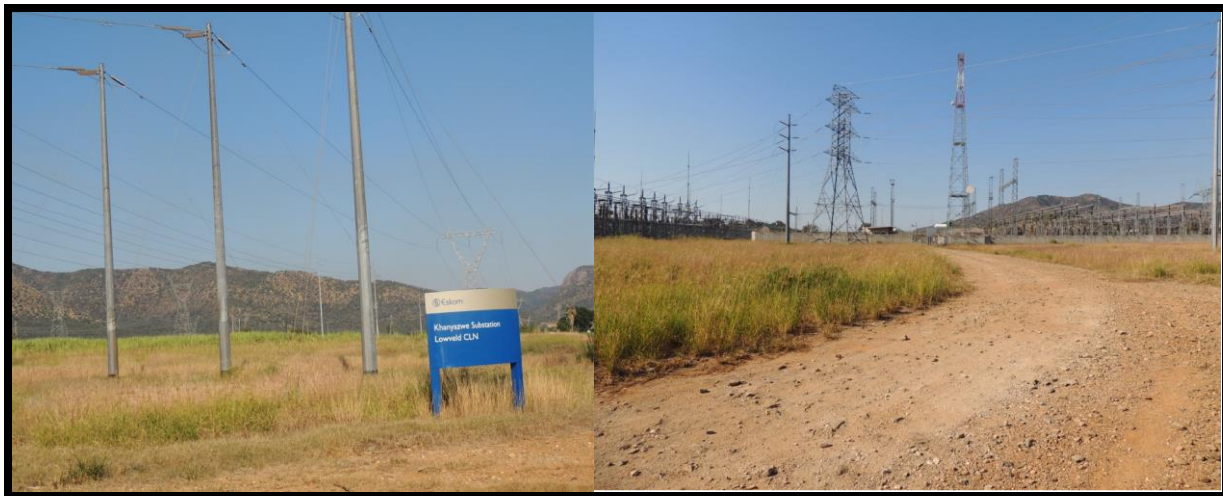
Figure 4: The power lines and substation within the proposed study area.
